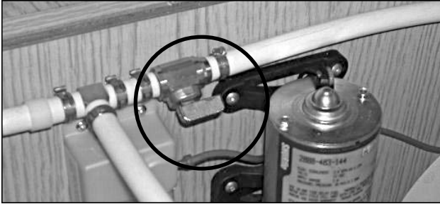
Picture G-P19: Hot water cutoff valve in open position.
